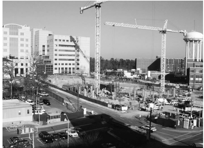
The University of North Carolina builds a new cancer hospital in Chapel Hill in February 2007.
